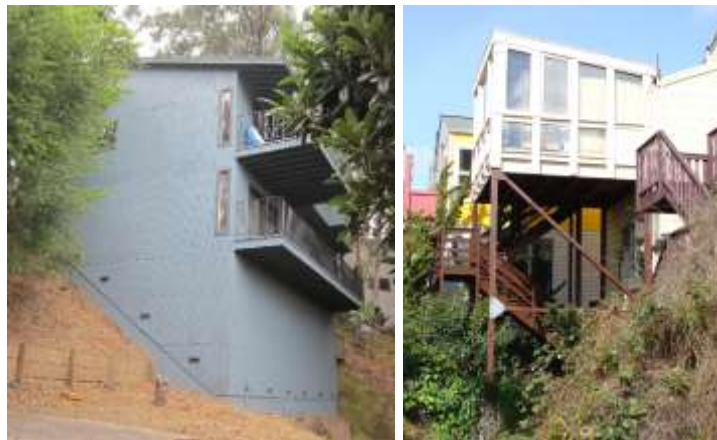
Figure 5-1 Hillside homes require special consideration; plywood shear walls perform badly in sloping walls as found in the house shown above left. Homes on steep sites can be very dangerous in quakes.
