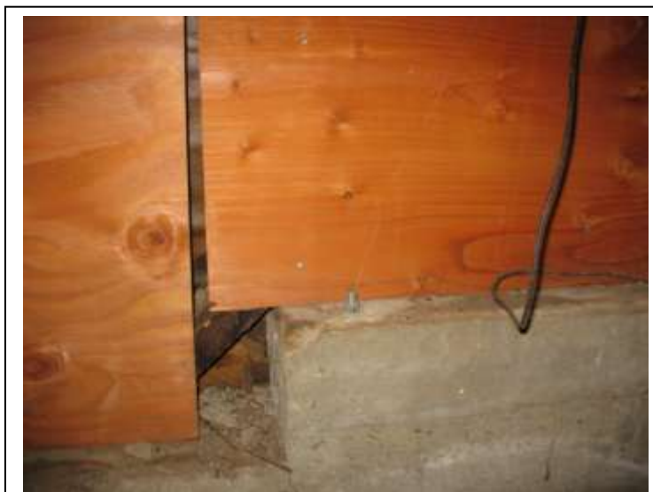
Figure 3-11 Plywood must be nailed to framing along each panel edge. TM—Max CamoW
