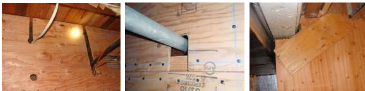
Figure 3-13 Slots severely weaken plywood bracing panels. If existing utilities cannot be avoided, slot length should be minimized (center) or a plywood patch glued to the plywood to reinforce it. The right-hand photo shows a diagonal patch that was installed to reinforce the notch at the upper-left corner of the plywood panel. © Paul R. & Thor M.
