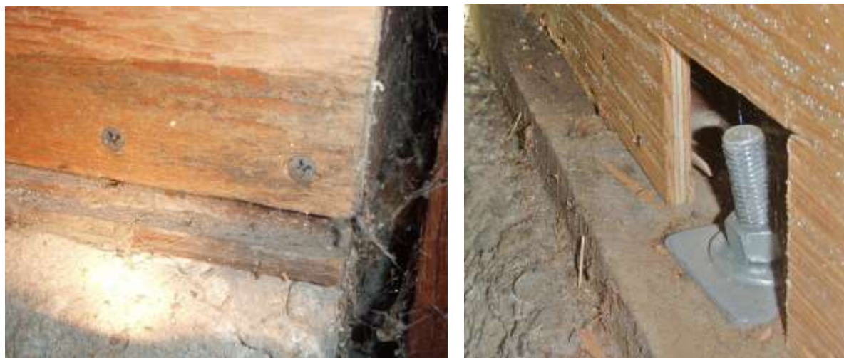
Figure 3-10 Defective plywood connections: Left—drywall screws; Right—toe-nails along bottom edge of plywood into the mudsill. TM-RDW, Mar C
