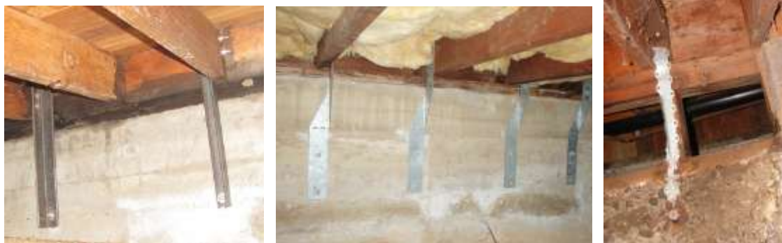
Figure 3-5 The steel angles, “hurricane ties” and flat steel straps shown are not appropriate connectors to resist earthquake forces.
