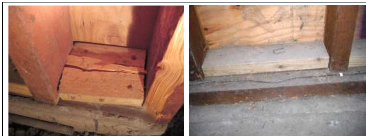
Figure 3-12 Mudsill block problems: Left—Split block; Right—lack of visible connection from block to mudsill. TM—Paul Rude
