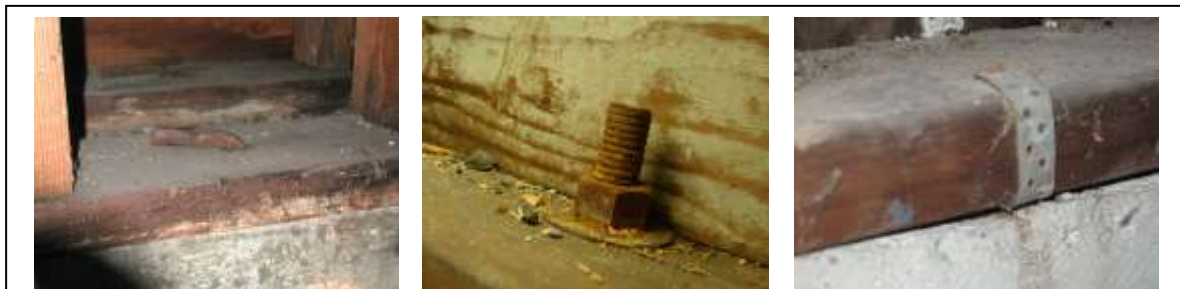
Figure 3-2 Mudsill connections used in the past. From left to right: Steel rod, pin, or bolt bent down over mudsill; bolt with standard round washer and nut; proprietary sheet-metal strap embedded in concrete and wrapped around and nailed to mudsill.
