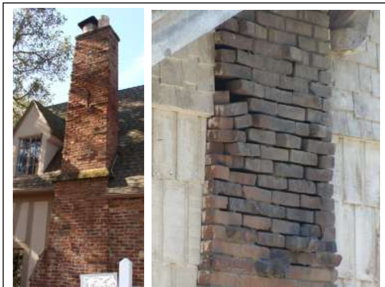
Figure 4-8 Chimneys are hazardous even when they are in good condition. Slamming the front door could cause the disintegrating chimney shown at right to collapse.
